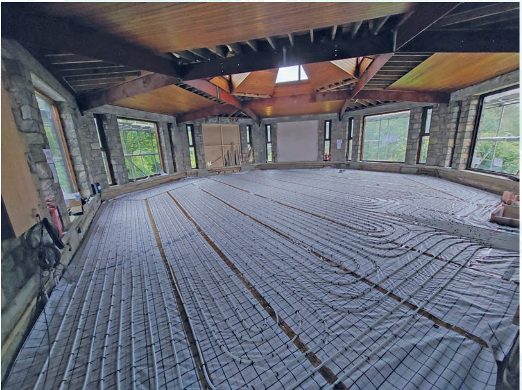
Underfloor heating in the Marsh Lounge
